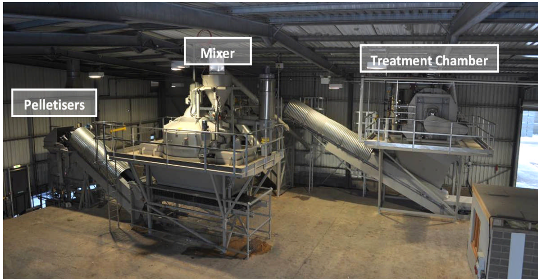
Figure 5. The newly commissioned plant
